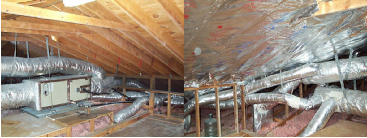
Figure E-3. Site #199 pre retrofit. Note attic air handler.
